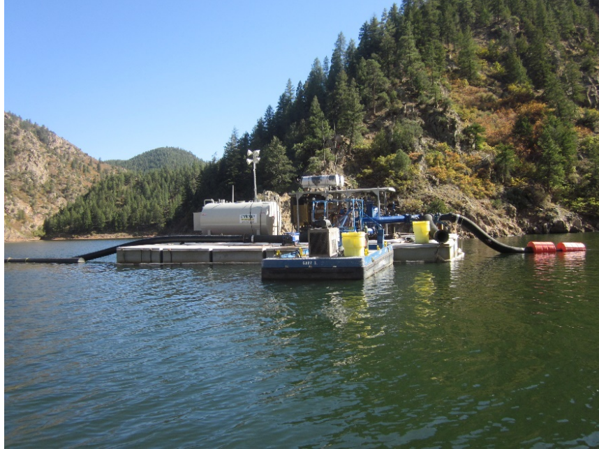
Figure 27. Floating sediment slurry pipeline and pumping plant on Strontia Springs Reservoir near Denver, CO (Photograph taken by Tim Randle, October 2011).
