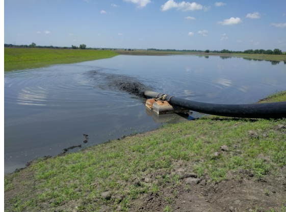
Figure 26. Dredged reservoir sediment being placed in a Confined Disposal Area at John Redmond Reservoir, KS.
